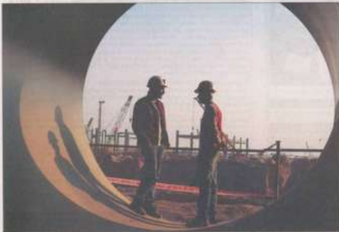
Work is in full swing to complete the first phase of the thermal power plant in Barwala village.
