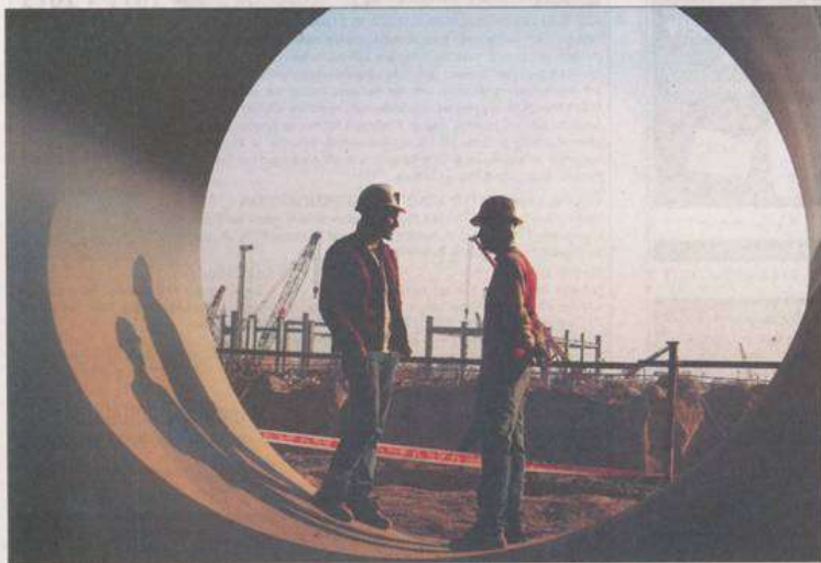
Work is in full swing to complete the first phase of the thermal power plant in Banwala village.
